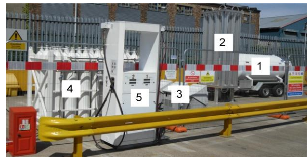
Figure 1: Temporary refuelling station showing (1) cryogenic storage tank (2) vaporiser (3) gas compressors (4) compressed gas storage (5) gas dispenser
